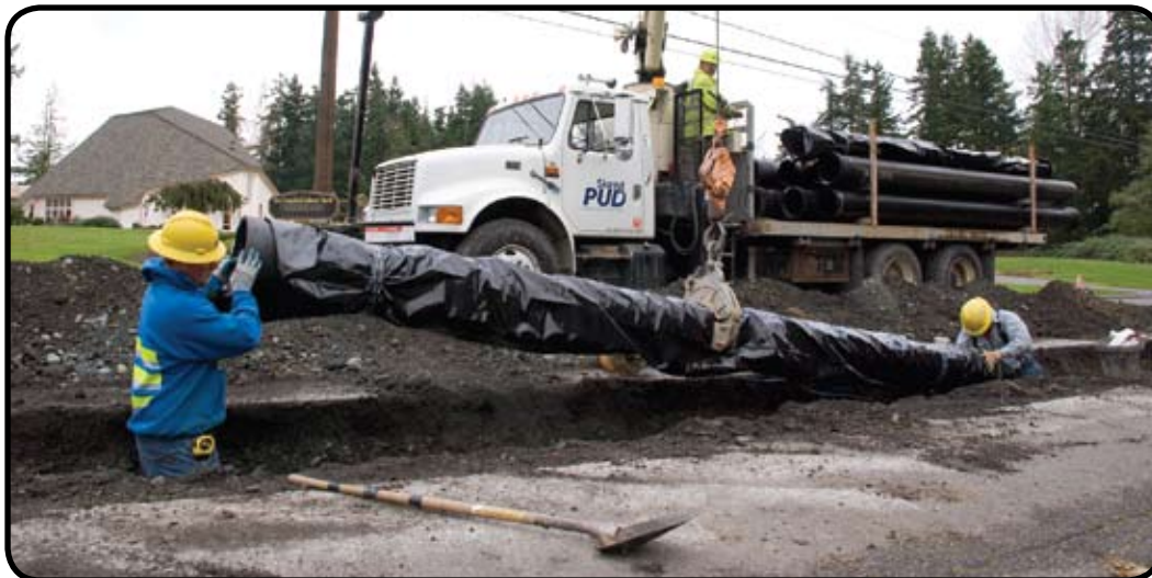
As part of Skagit PUD's ongoing capital improvement program, crews recently replaced 1,420 feet of six-inch asbestos-cement pipe with 12-inch ductile iron along Blackburn Road in Mount Vernon.
