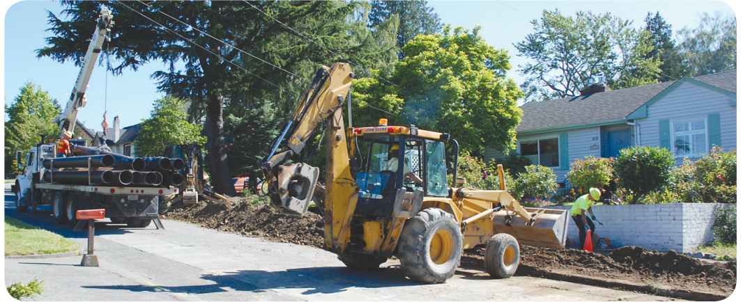
Skagit PUD crews install a new section of 12-inch water main on 9th Street in Mount Vernon as part of our ongoing capital maintenance program. Several new projects are slated for this summer including: 1,500 feet of water main replacement in Clear Lake; installation of test wells to check groundwater levels along Josh Wilson Road; and a new pump station near La Conner.
