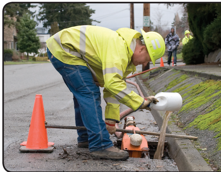
Water quality worker Ryan Anderson checks for sediment in a water line as part of Skagit PUD's ongoing flushing program.
