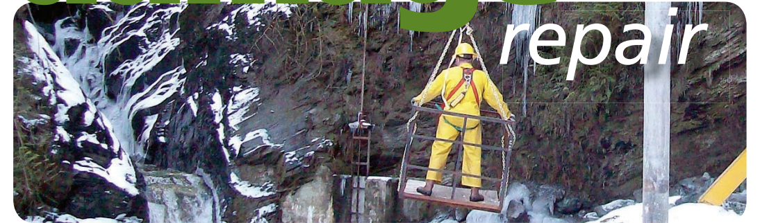
A PUD construction worker takes a closer look at storm damage at the Gilligan Creek water supply intake.
