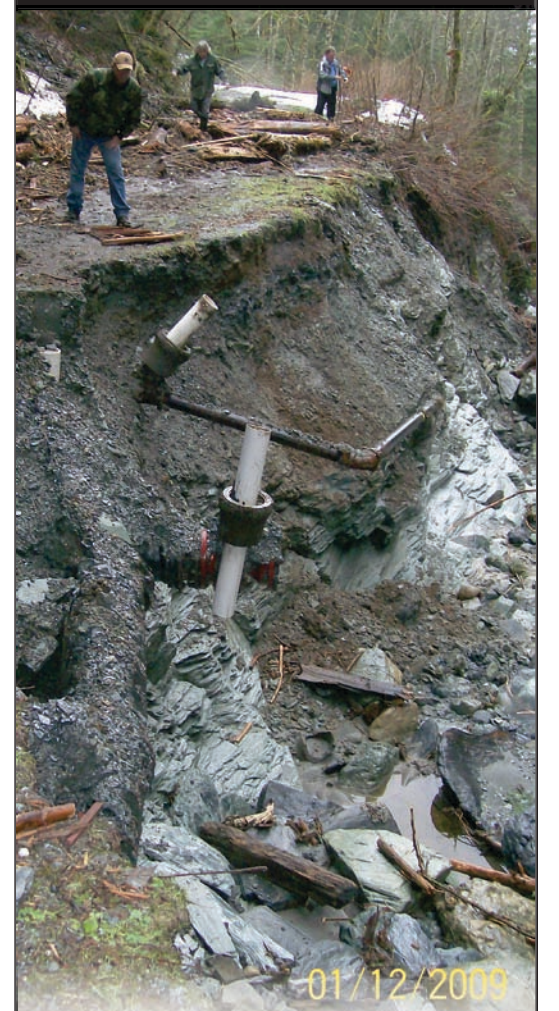
(Above) PUD staff inspect severe bank erosion at our Gilligan Creek intake site. Gilligan Creek is the source for 70-percent of the PUD's water supply.
