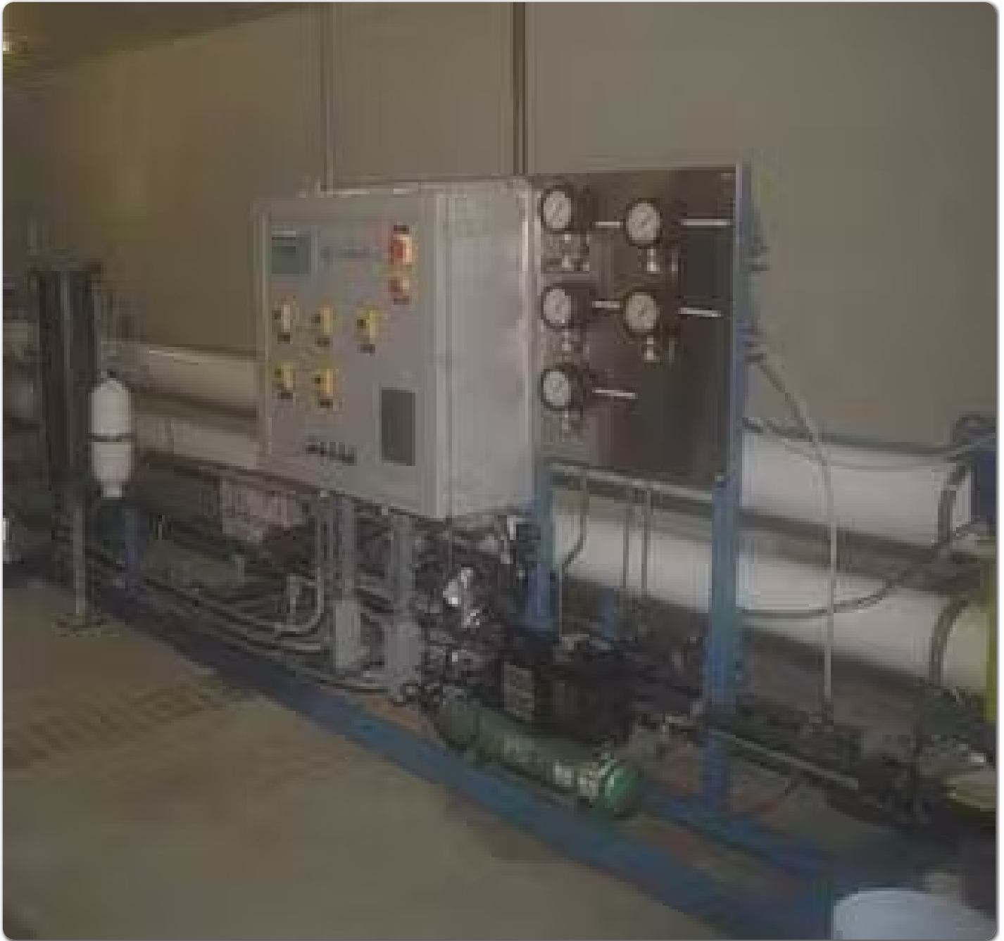
The MUNI RO system from Osmonics meet water supply requirements. Photo by Osmonics
