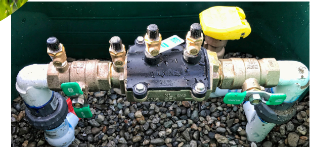
DCVA in a below-ground enclosure.
